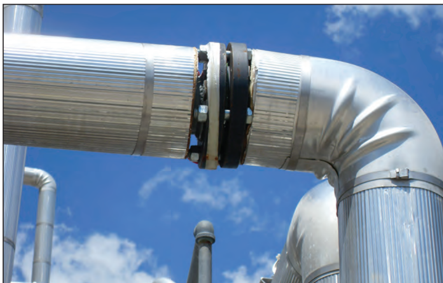
FIGURE 3. Pipe flanges are potential sources of leaks. Design considerations are important here
